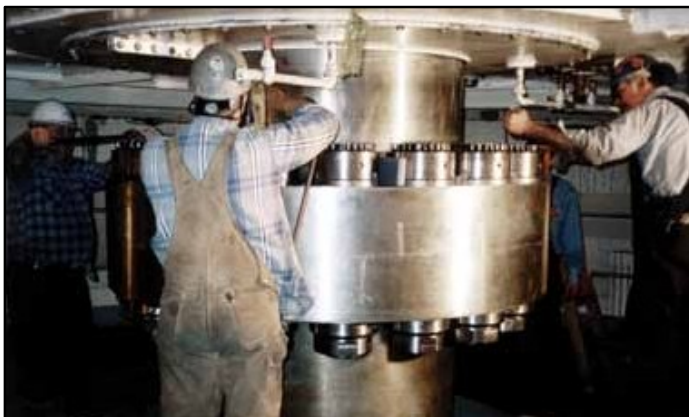
Kaplan turbine coupling, (18) 6-3/16" studs. The previous method required 150-250 man hours utilizing a 150 lb. "dead man", a 50 ton hydraulic ram, and a 250 lb. wrench. Supernuts® were installed in 2-1/2 hours using 1/2" air impacts and hand torque wrenches.
