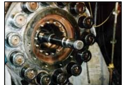
Ingersoll Rand boiler feed pump with 6" diameter studs (H650TX-600-8/w). With air tools, tightening required only 2-1/2 hours.
