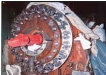
Boiler feed pump rebuild utilizing Superbolt® H650X Tensioners.
