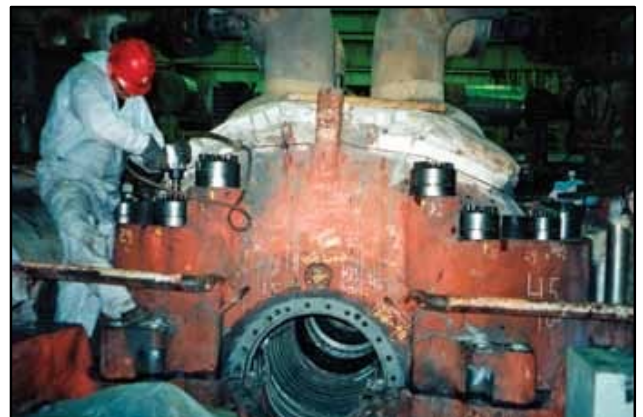
MT Supernuts® used as a closure tool. The shell had to be bolted up without the rotor assembly for measurements. The tensioners were used to speed up the maintenance schedule thus saving valuable outage time. Supernuts® are reusable for repairs on other turbines within this utility.
