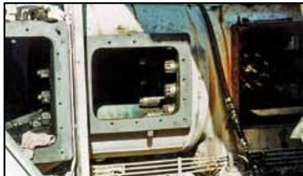
Reciprocating compressor, distance piece.
