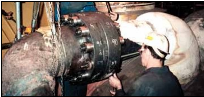
High pressure steam lead with rotational misalignment of bolt holes. Solved leakage and history of bolt failures.
