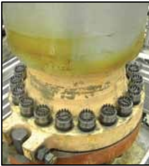
Main steam inlet flange.
