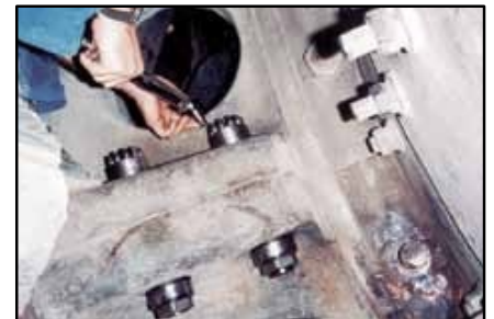
Split Gear segment on rotating kiln.
