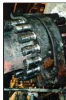
High pressure steam turbine inlet flange.
