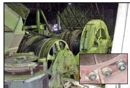
Hoist and drag drums.
