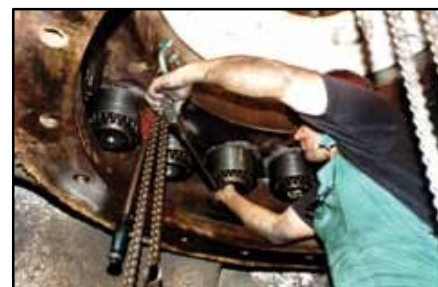
Overhead work is simplified with the low torque requirement on this Turbine Wheel to Shaft bolting. Galling and seizure is eliminated.
