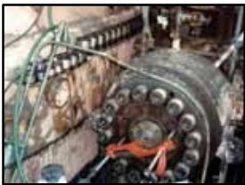
HP turbine and valve
