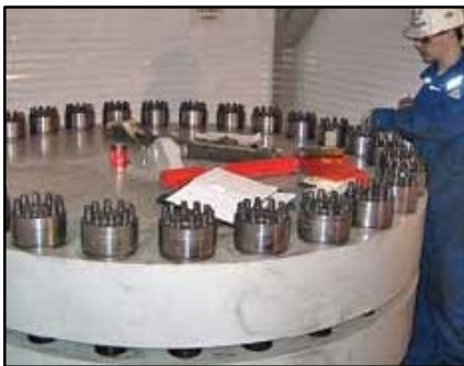
Compressor inlet filter cover.
