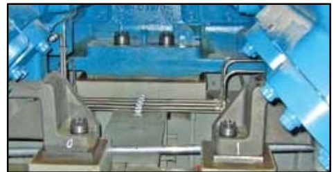
Anchorbolts on crank case and distance piece of a compressor.
