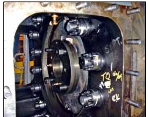
Our products are especially useful in limited space applications, such as this distance piece on a reciprocating compressor.
